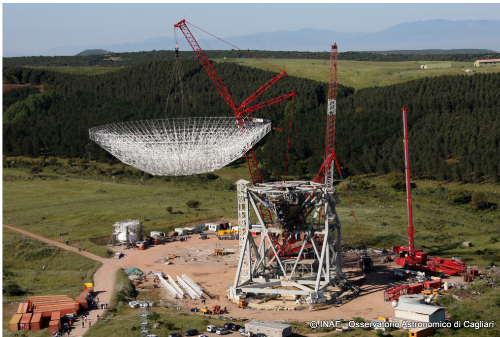
Fig. 3. It is 22nd May 2010, it is the day of the "big lift": one of the largest European cranes is used to bring the rib structure that will support the primary mirror of the radio telescope to the top and place it on the alidade. Another public event, great technological success resulting from courageous choices: this is Nichi.
